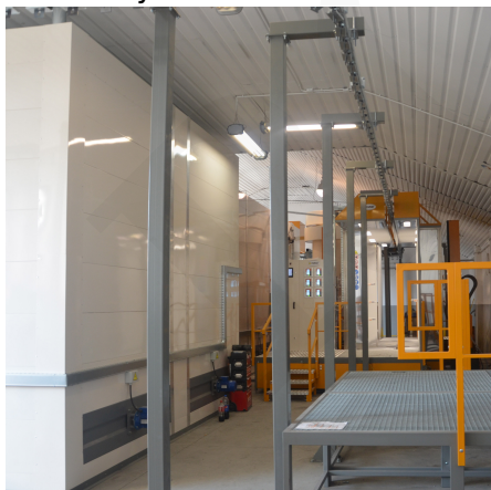
Suspended chain conveyors
